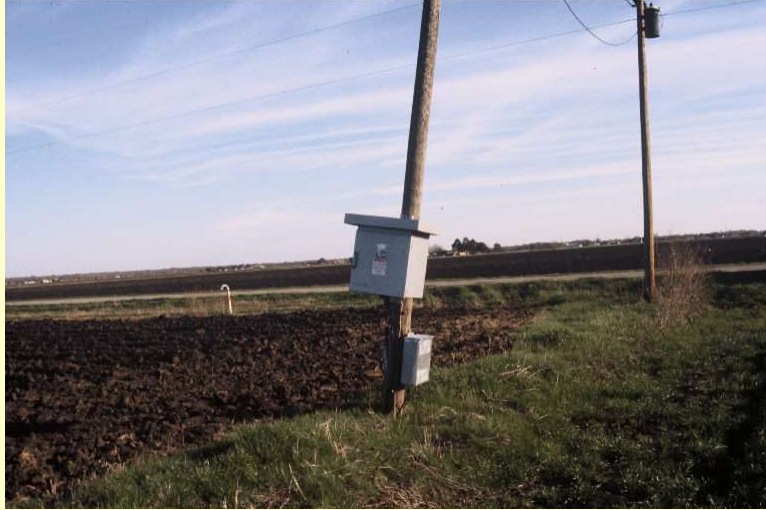
Pole about to fall over. Should correct before failure
